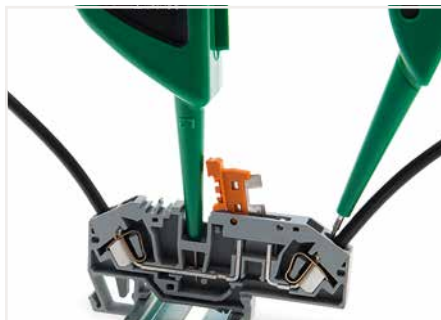
Testing via jumper contact slot.
