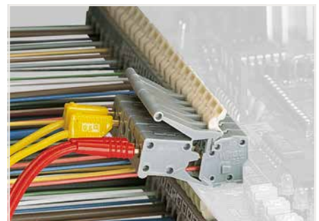
Testing with test plug modules.
